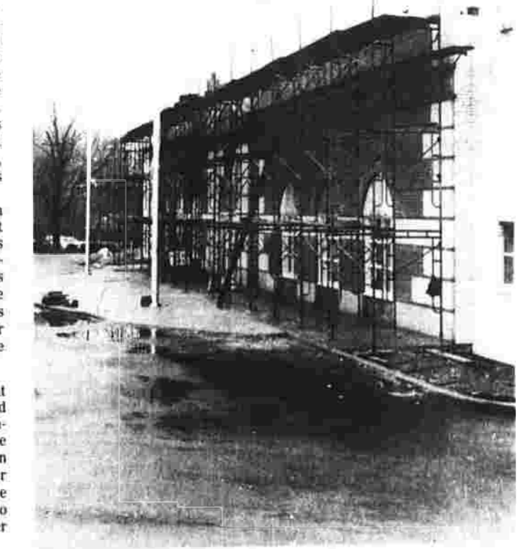
Work continues on the new Manchester Superior Court at the intersection of Center and West Center streets. The new facility is scheduled to open in June. (Herald photo by Foley)
